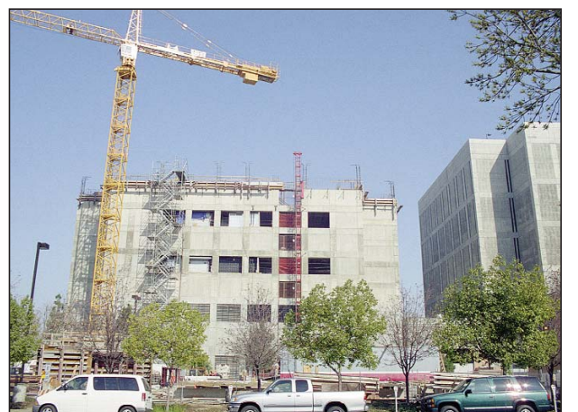
Construction of the expansion to the Fresno County Jail to include Criminal Court Departments 95 & 96.
